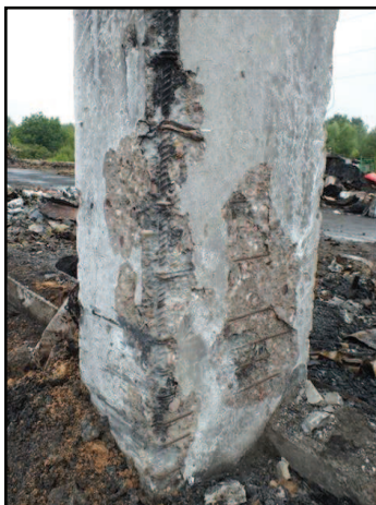
Figure 4: Peeling of crumbly protective layer of concrete, visible reinforcement
