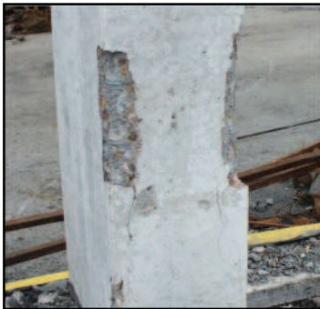
Figure 3: Cracking, separation and peeling of concrete along the column edges (up to the main longitudinal reinforcement), pronounced change in aggregate colour, net-like fissures
