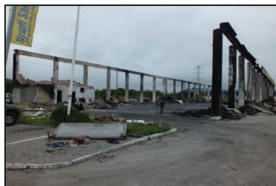
Figure 2: Object's appearance after fire and clearing the ground off
