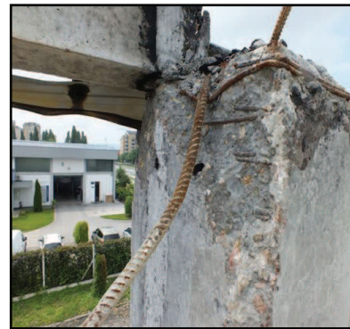
Figure 6: Crumbling of concrete in the supporting zone, peeling of surface and protective concrete layers, deformed stirrups and anchors, change in aggregate colour
